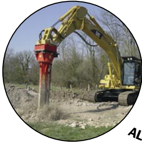
ALLU PM Power Mix - mixing soil and binding agent in mass stabilization
